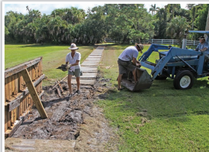
Time is taking a toll on the Smith Mound Boardwalk. Lee Tapager, Patrick Rennert, Charles O'Connor (not pictured), and Mark Chargois completed a temporary repair; however, a complete replacement will be required in the near future. Sponsorship of the boardwalk repair is available by contacting Cindy Bear or Bill Marquardt. (Photo by C. O'Connor.)
